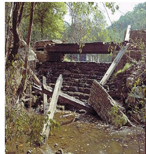
Damaged historic dam
