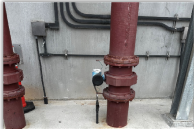
Influent pump station discharge piping.
