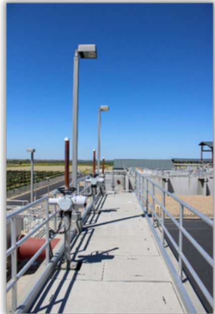
Light fixtures at the Water Recycling Facility.
