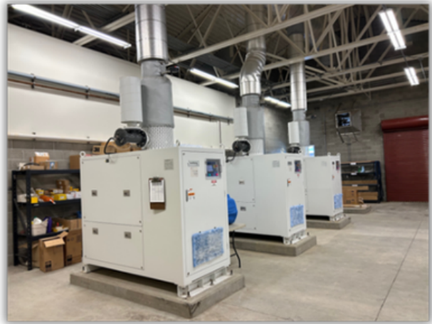
Aeration blowers for Membrane Bioreactor.
