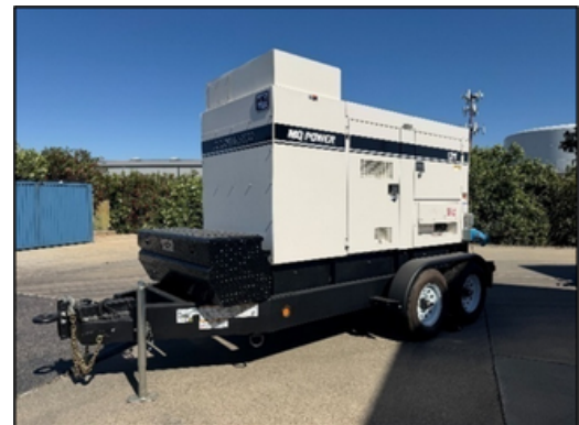
Generator used for emergency power outages.
