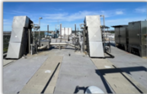
Influent pump station headworks.
