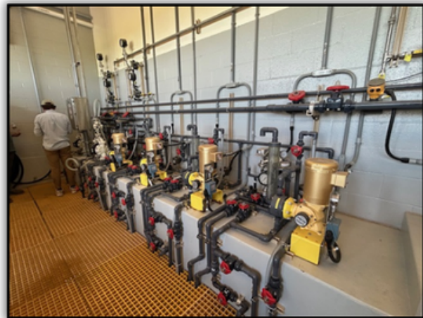
Chemical pumps and feed lines.
