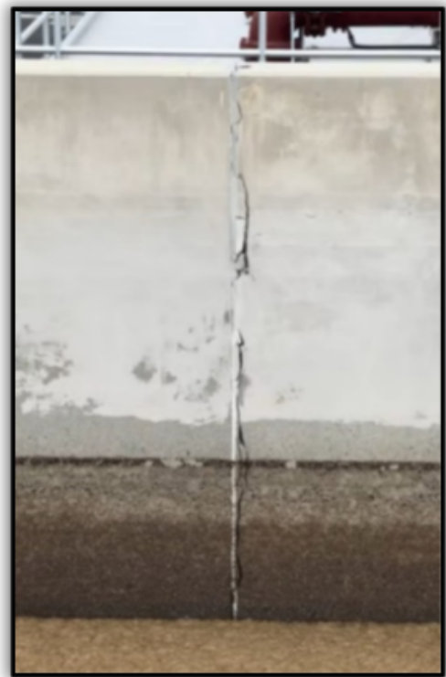
Structural crack at aerobic digester.
