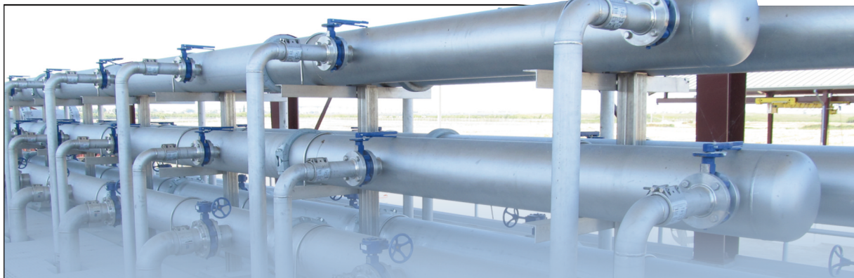
Hidden below these steel tubes at the ISD Water Recycling Facility are hundreds of microfiltration membranes like the one seen below.
