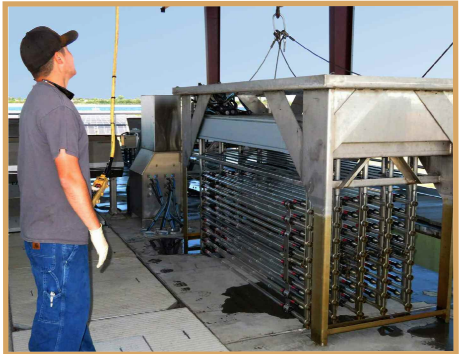
Inspecting ultraviolet light system at the Water Recycling Facility.
