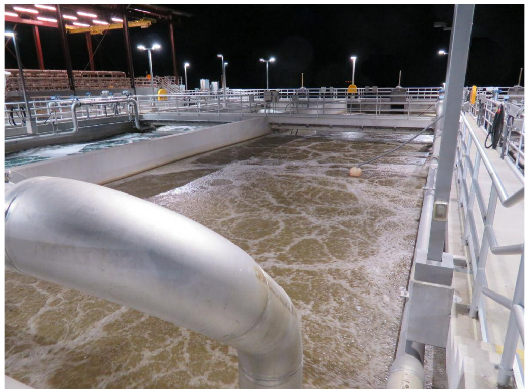
Aeration Basins at Ironhouse Sanitary District's Water Recycling Facility.
